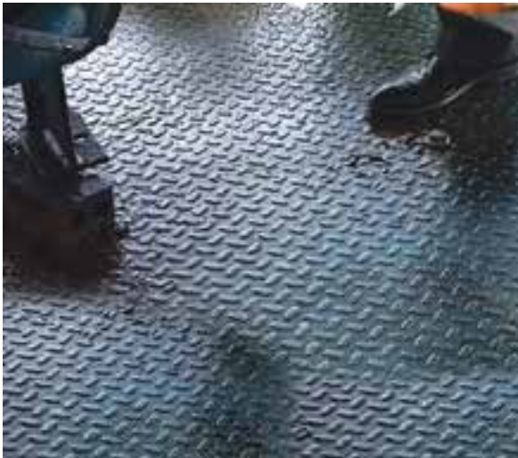
1. The floor is stained with oil
