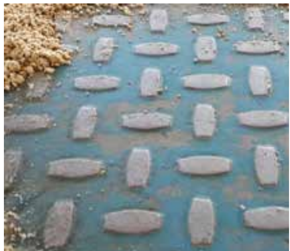
4. The floor is clean, no oil left
